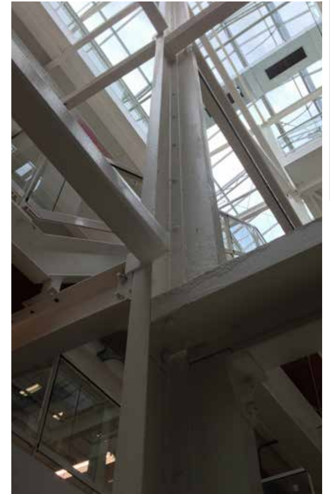
Figure 4. Connecting the old and new doesn't always fit exactly.
